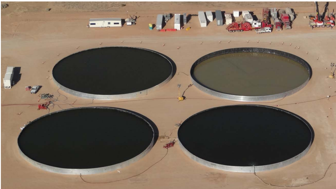
Figure 10: Above Ground Storage Tanks, Cowralli Multi-well pad, Cooper Basin 2013
